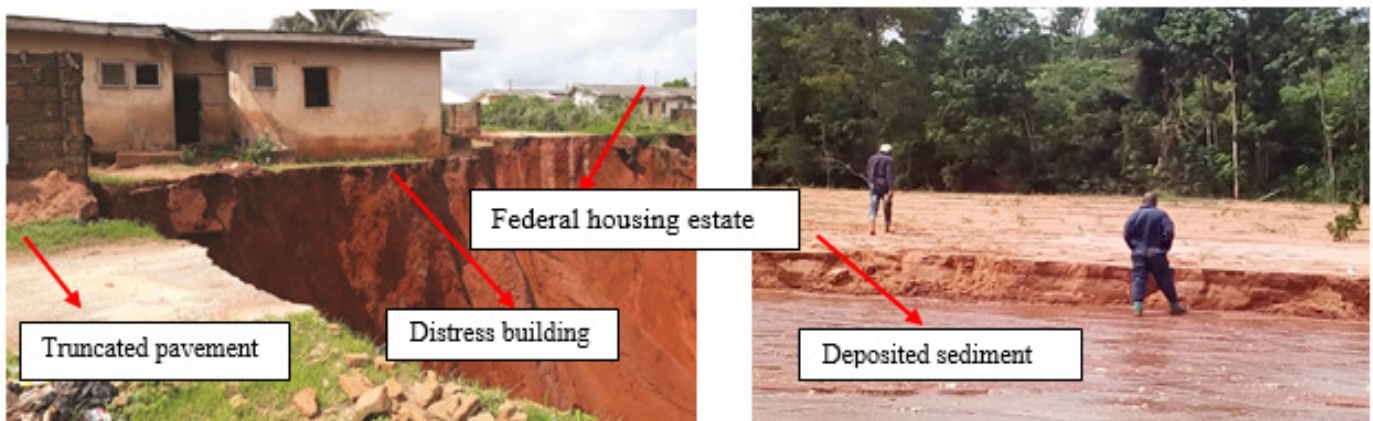
Figure 3. Devastating impact and soil loss from Gully B
